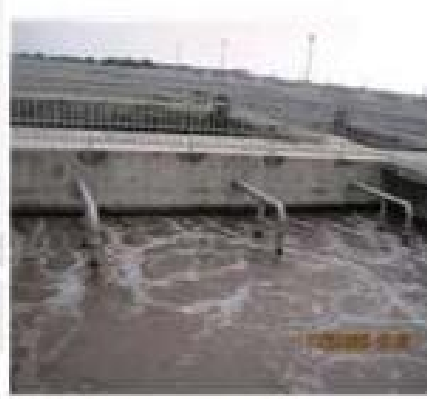
Aerated tank Binh Hung Waste Water Treatment
